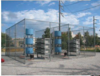
A completed 11 kV 5 Mvar bank
