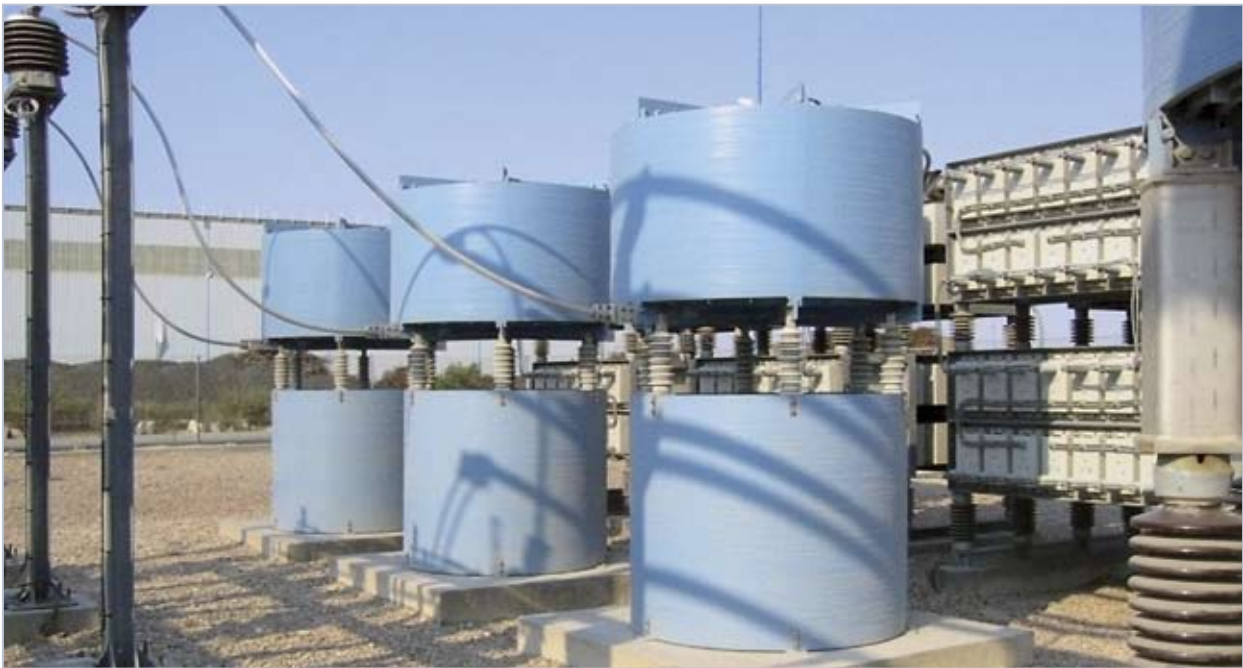
130 Mvar, 30 kV, 50 Hz, Sonasid, Morocco
