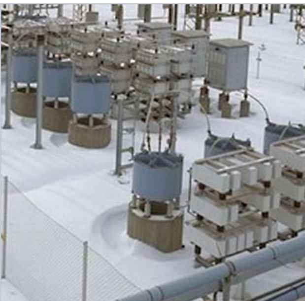
A 130 Mvar / 21 kV-50 Hz SVC installation at the Outokumpu Polarit steel plant, in Tornio, Finland. The filter banks and thyristor controlled reactor are located in the outdoor switchyard, while the thyristor valves, control and protection system and switchgear are located inside the pre-assembled building in the back.
