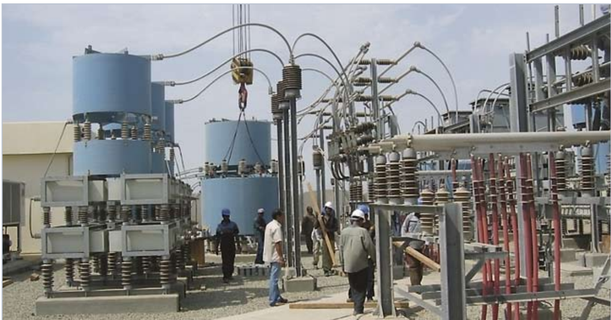
130 Mvar, 30 kV, 60 Hz, Rajhi Steel, Saudi Arabia
