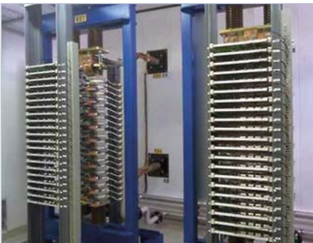
OUTOKUMPU POLARIT, Tornio Finland SVC 130 Mvar, 20 kV 50 Hz
