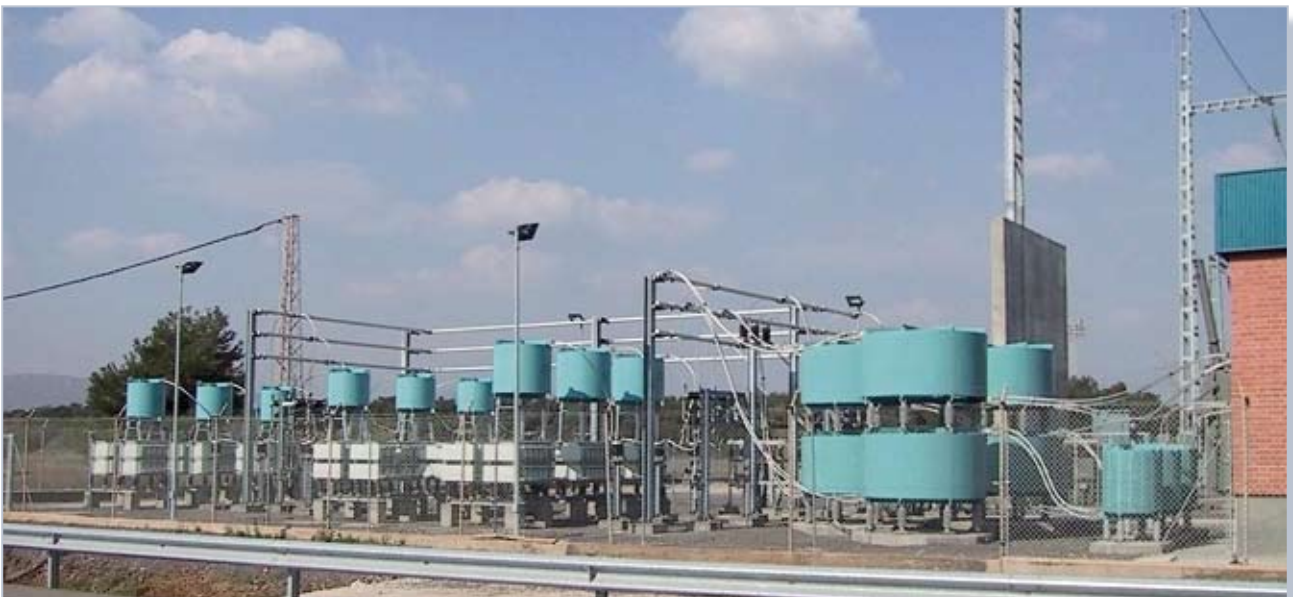
Sidmed, Spain SVC 65 Mvar, 20 kV, 50 Hz
